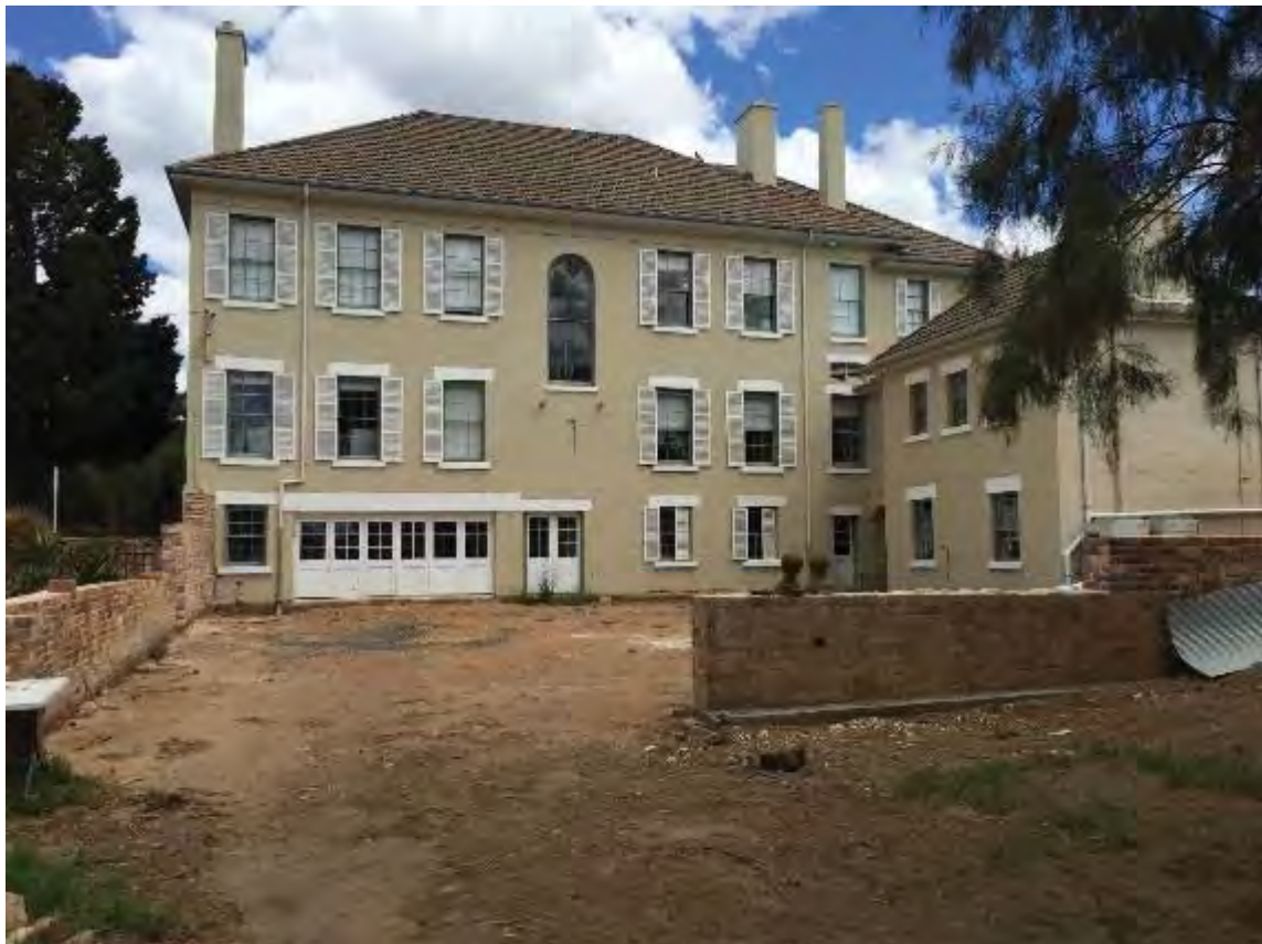
Figure 69: Current Oct 2017 view of the rear (north elevation) of the property. Note the rear courtyard brick wall had gone past the safe lean point and had been assessed by a structural engineer as unsafe and had to be carefully dismantled for safety reasons. TTA Oct 2017
