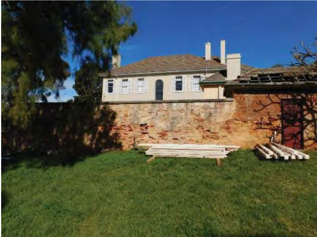
Figure 68: The rear brick wall surrounding Oran Park House showing its poor condition. TTA 2013
