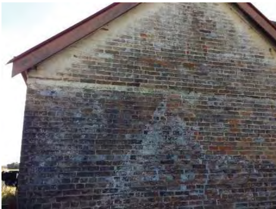
Figure 144: Original south wall of the coach house. It is suggested this is the original house c1837. TTA 2013
