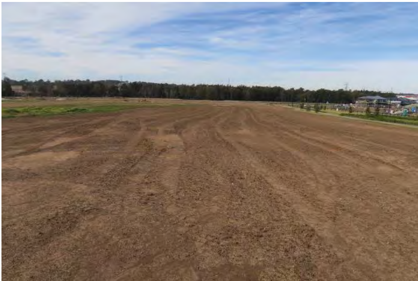
Figure 105: Grading of the land in the southern portion of the site looking to the east showing the fringe of surrounding residential subdivision development. Source: Casey & Lowe: 2017: pg.13, Figure 3.4.
